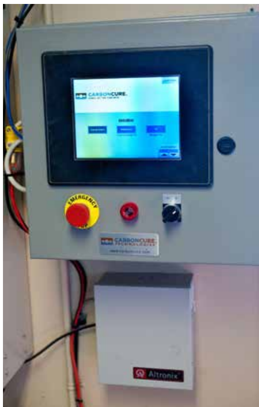
Thomas Concrete/Doraville staff can operate the CO 2 injection system on a touch screen panel integrated with the batch control system.
